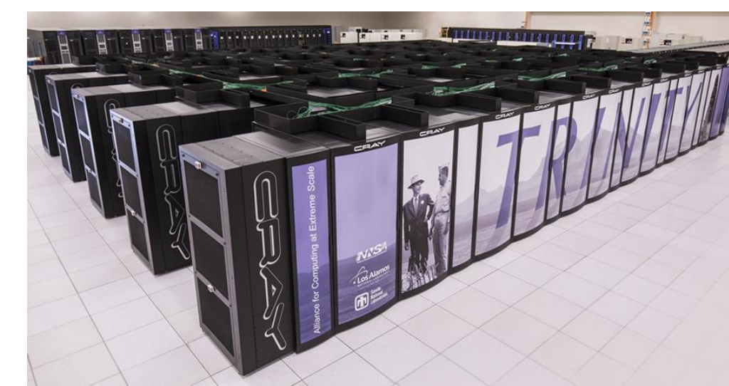
Trinity, a supercomputer at LANL, with almost 20,000 compute nodes and 78PB of capacity.
